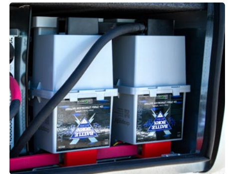
Additional Smart Lithium Battery 270-Ah 12-V with Internal Heating System (540-Ah total)
