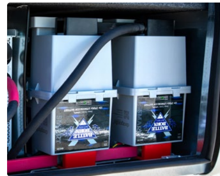
Additional Smart Lithium Battery 270-Ah 12-V with Internal Heating System (540-Ah total)
